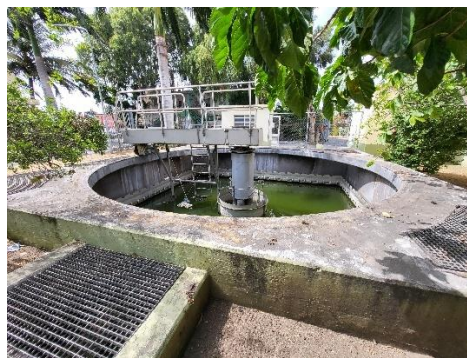
Photo 2-3 – Primary settling tank
