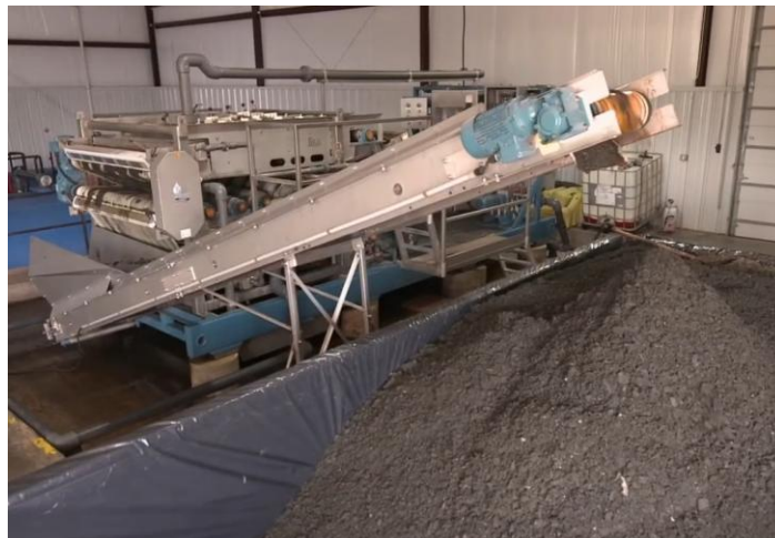
Figure 7-1 – Discharge of the mechanically dewatered sludge to a container 105
