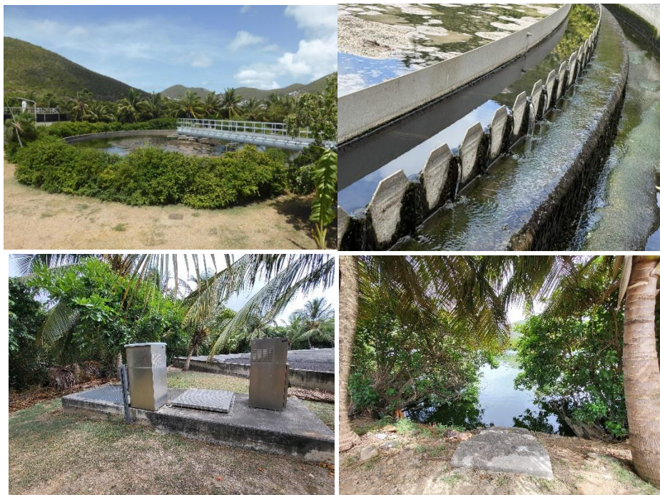
Photo 2-7 – Secondary settling tank, with purified water (top photos) and control system before the discharge at Fresh Pond (down photos)
