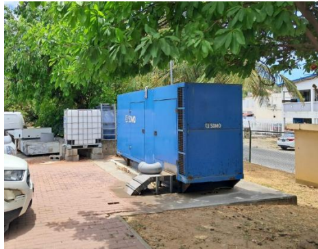
Photo 2-15 – Power generator and diesel tank
