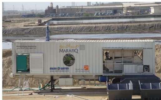
Figure 2-7 – Sludge treatment equipment (New mechanical dewatering system belt filter)
