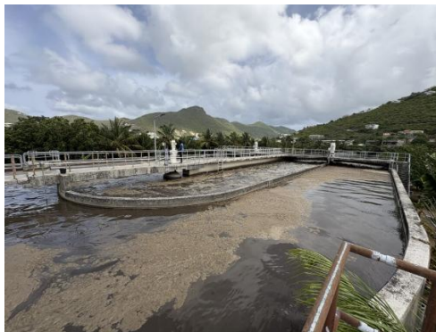
Photo 2-5 – Aeration tank with the biologic reactor
