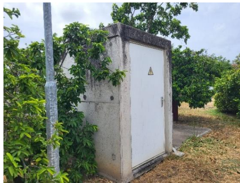
Photo 2-11 – Sludge pumping station
