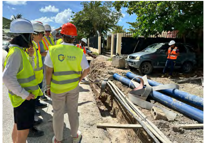
Crews installed underground electricity distribution lines with NV GEBE, strengthening the island’s power network and safeguarding crucial services during extreme weather.
