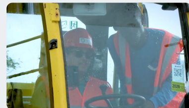
▶ Demolition of the Old Library Building Paving the Way for a Modern Future
