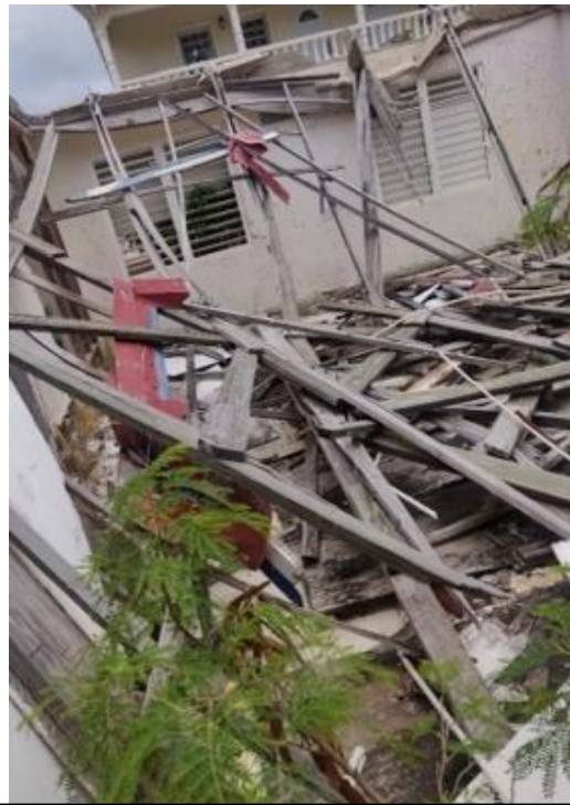
Destroyed classroom beyond repair at CLB
