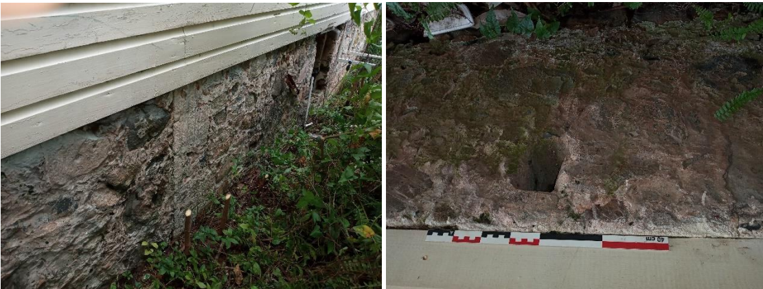
Figure 11. Feature B main building historical sub-floor foundations; (upper left) exterior access opening on the west side; (upper right) interior view; (lower left) north extension discontinuity with older foundation wall, and (lower right) drain opening in north extension, which may indicate it was formerly used as a cistern.
