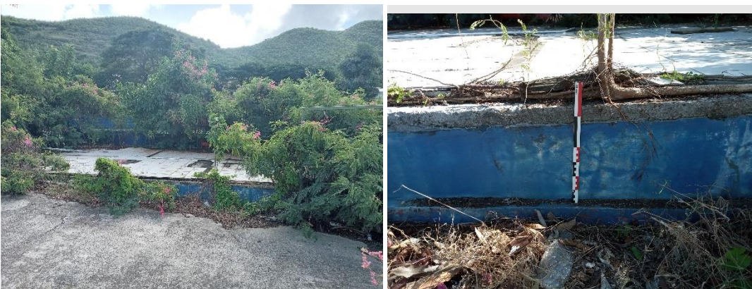
Figure 9. Feature B, being a reduced foundation structure at the CLBS property, these are all that remains of the former police watch-post.
