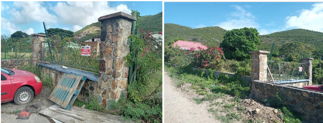
Figure 8. Entrance Gate structure (Feature A) at the CLBS property (post-1916). Also seen with original full entrance in Figure 2.
