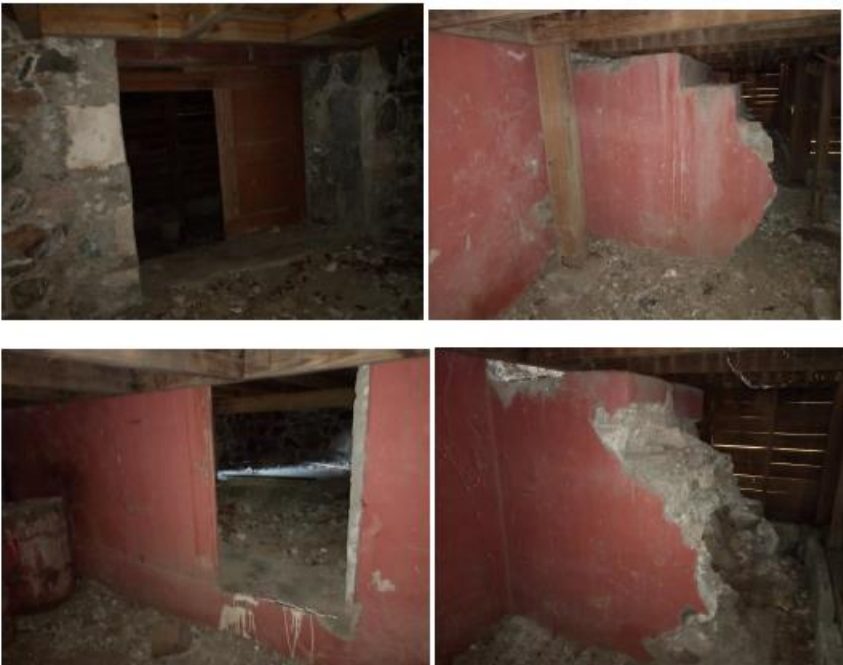
Figure 10. Feature B, Main School Building historical foundations, located beneath the floor beams of the new front porch, with two front steps and a shuttered opening.
