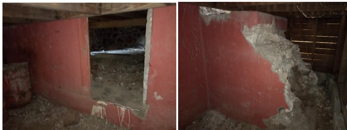
Figure 12. Feature B, Main School Building historical foundations, located beneath the floor beams of the new front porch, with two front steps and an intact shuttered opening.
