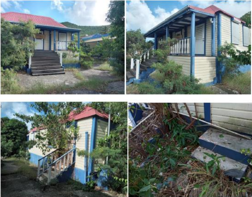
Figure 8. Modern restored Main Building structure above Feature B; (lower left) new steps on the east side, (lower right) the two new steps at the north side.
