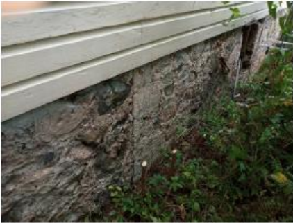
Figure 9. Feature B main building historical sub-floor foundations; (upper left) access opening on the west side; (upper right) interior view; (lower left) north extension discontinuity with older foundation wall, and (lower right) drain opening in north extension, which may indicate it was formerly used as a cistern.
